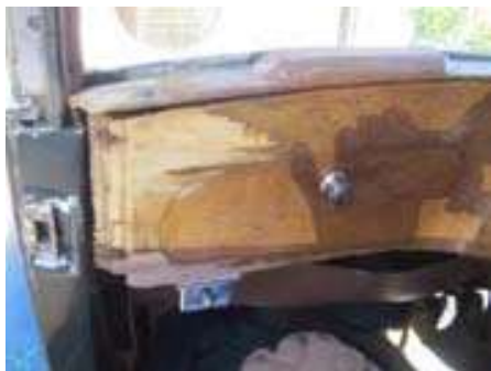
An extreme example of decay!
