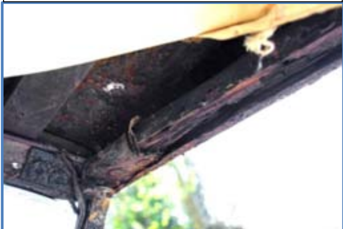
Leaking gutters leading to rotten wood and metal
