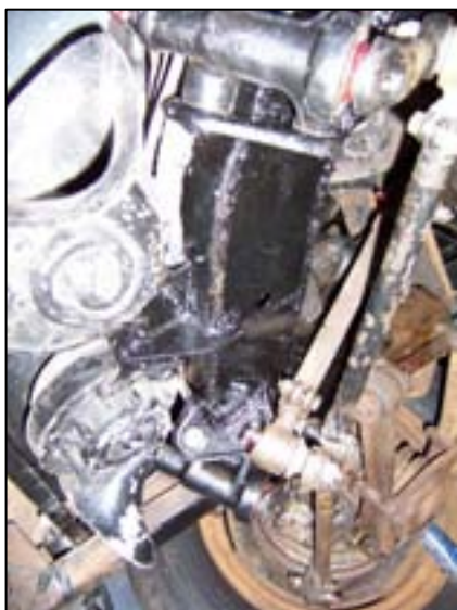
The front cross-member once welded up and painted, seen from under the front of the car.
