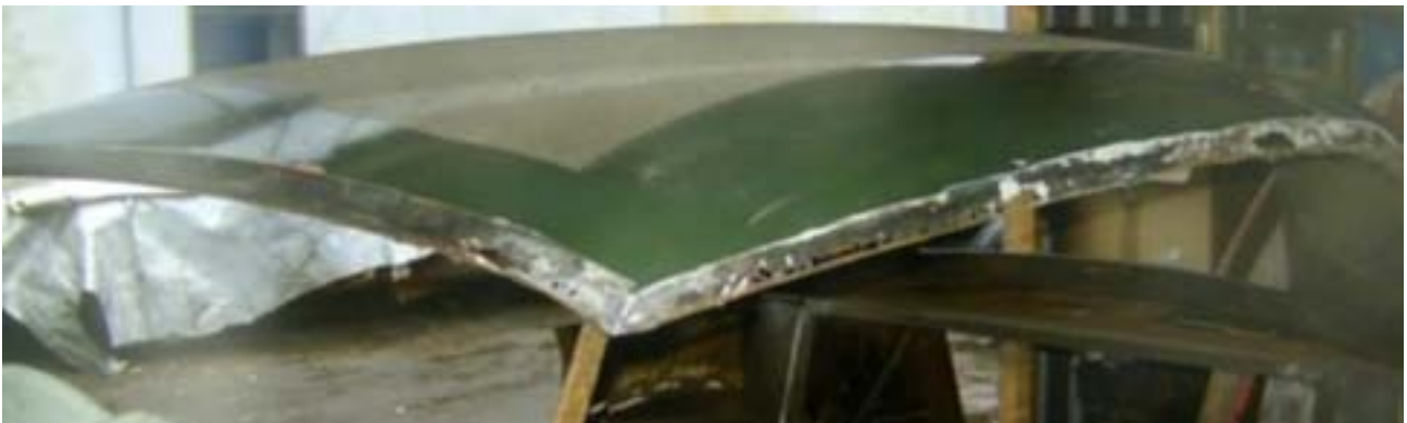
Exposing and cleaning the edges of the roof where holes need to be repaired.
